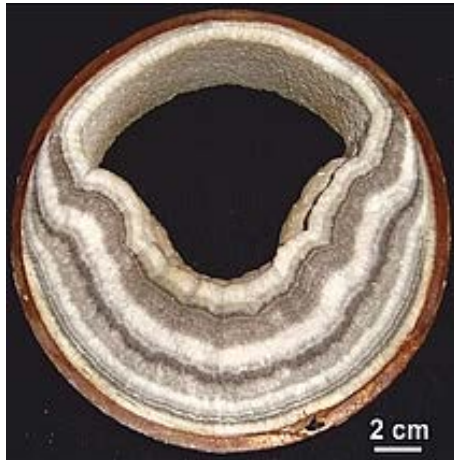
Rohrscalings © TU Graz
